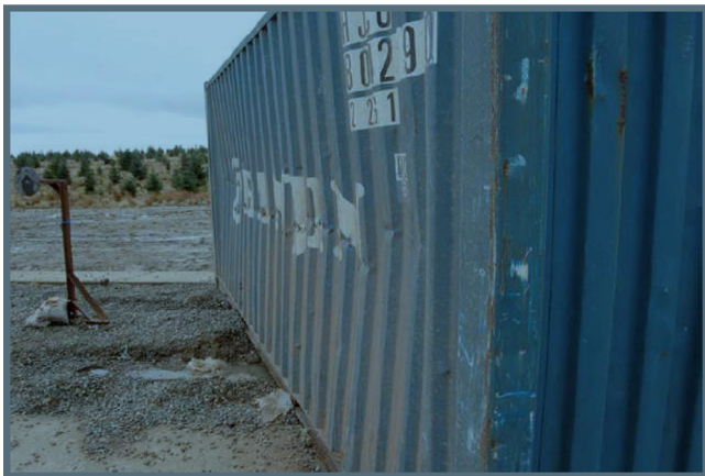
Fig. 19. Damage to an isocontainer when the incident overpressure was 2 atm (photograph reproduced from [33,34]).
